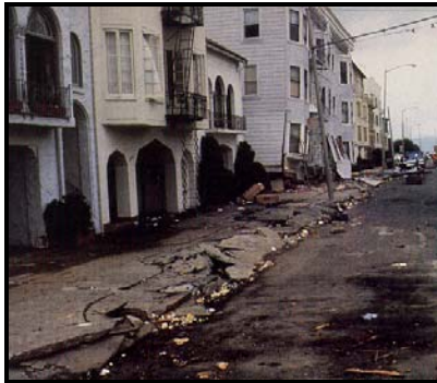
Liquefaction damage, Marina District, 1906 Loma Prieta, California, Earthquake Source – M. Bennett, U.S. Geological Survey
